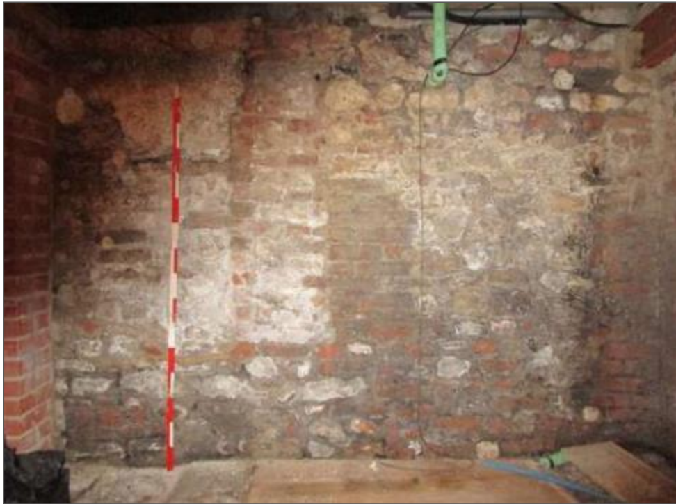
Plate XXIII: West wall of North cellar. Proposed door opening marked with red dashed line.
