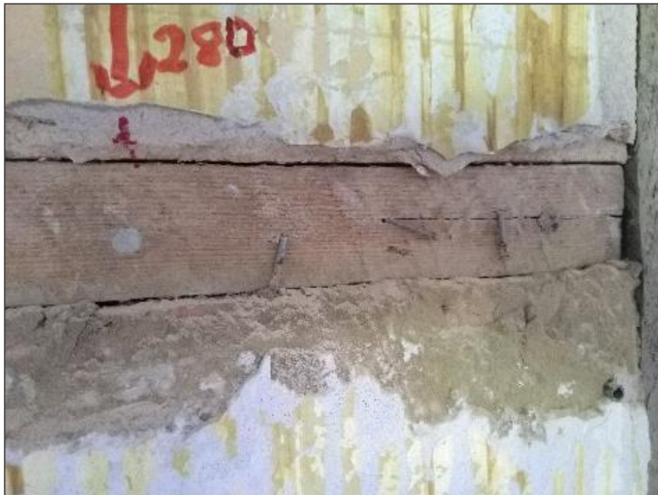
Plate VI: Modern infill to historic door opening Regularised timber rail with wire-cut nail fixings. Associated carlite plaster, brick and blockwork infill with cement mortar.
