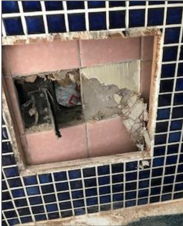
Plates III: West external wall - To be removed to enable proposed Bathroom extension 200x200mm Sample area of fabric removed - all noted to be mid-late C20.
