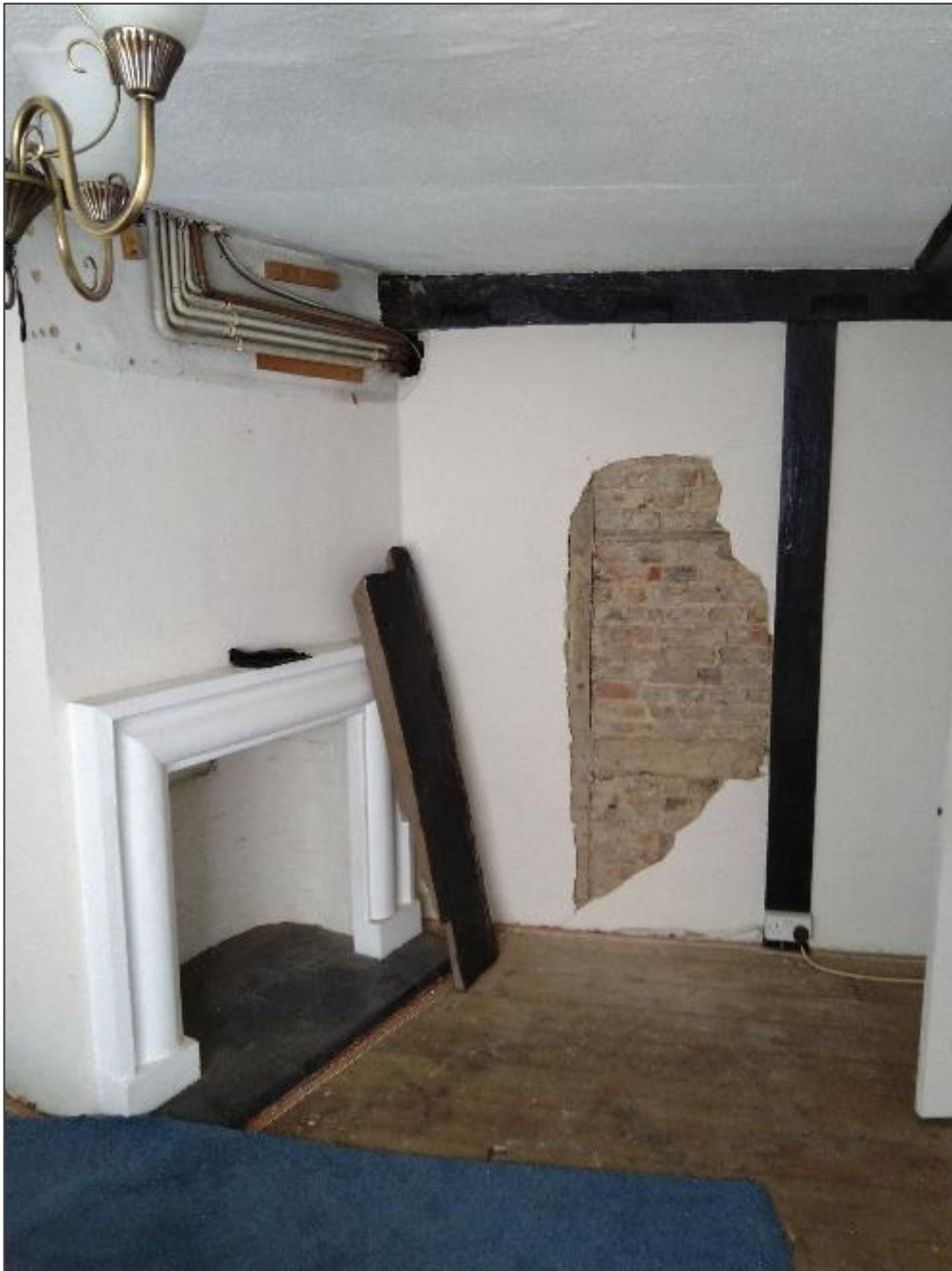
Plate XII: West wall of South Bedroom with area of modern cement plaster removed. Re-used C16 timber over proposed door opening.
