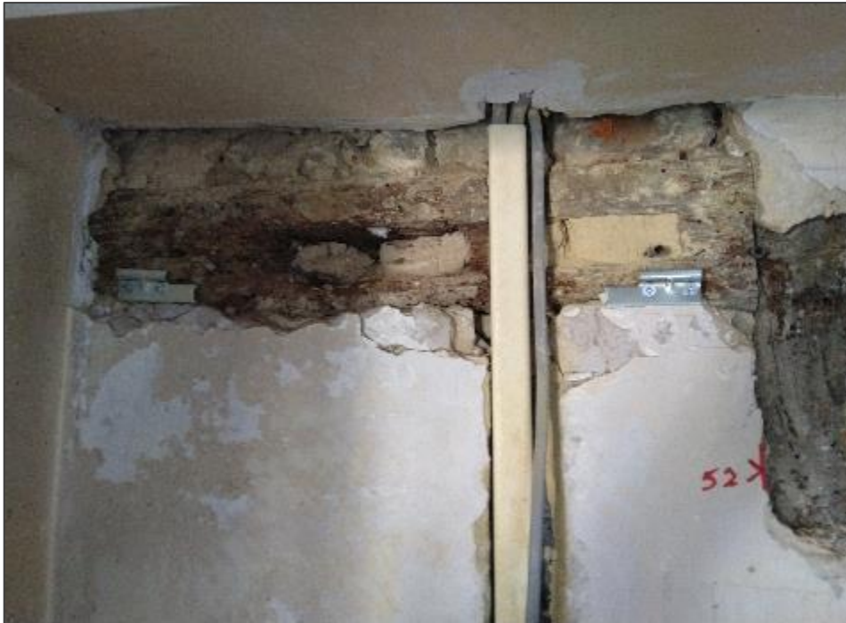
Plate VII: North end, Re-used C16 timbers with concrete blockwork infill beneath. Hollow mortice is associated with a vertical post and diagonal brace (timber not in-situ).
